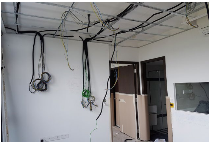
KNX bus cables are laid together with electrical wires.
